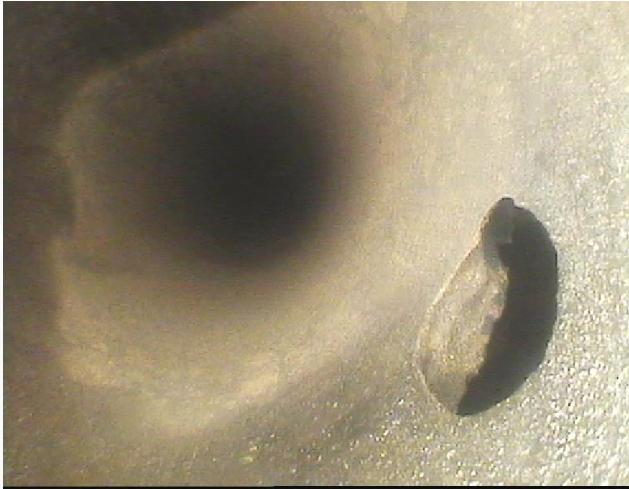
Fig 1: Leakage at 9.66m in R[1]C[1]
