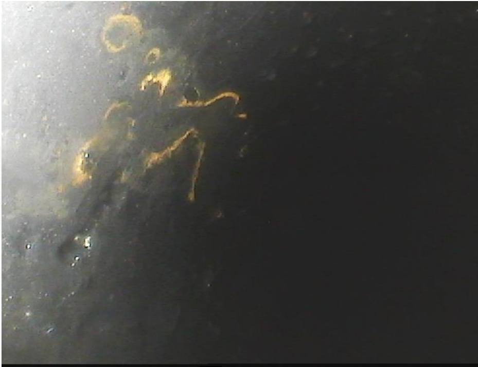
Fig 3: Wall loss at 8.15m in R[7]C[12]
